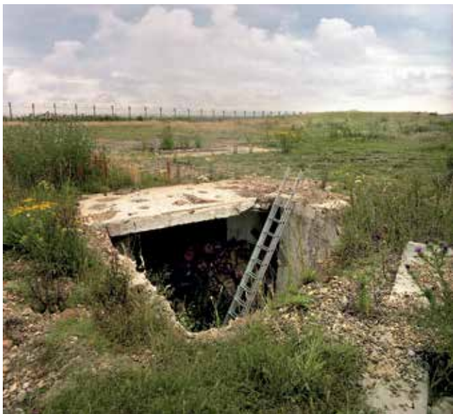
The excavated stairwell seen during the Sub Brit visit in July 2002. Photo Nick Catford
